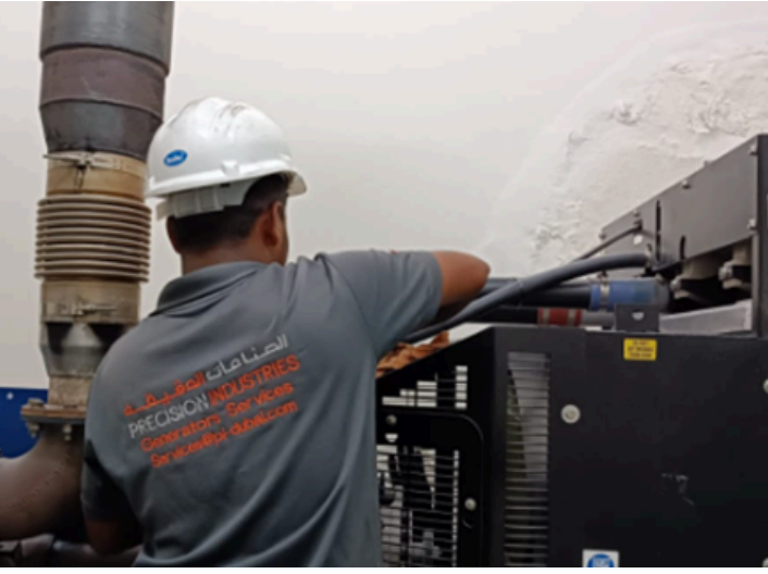
Generator Maintenance and AMC for more information - page 2
